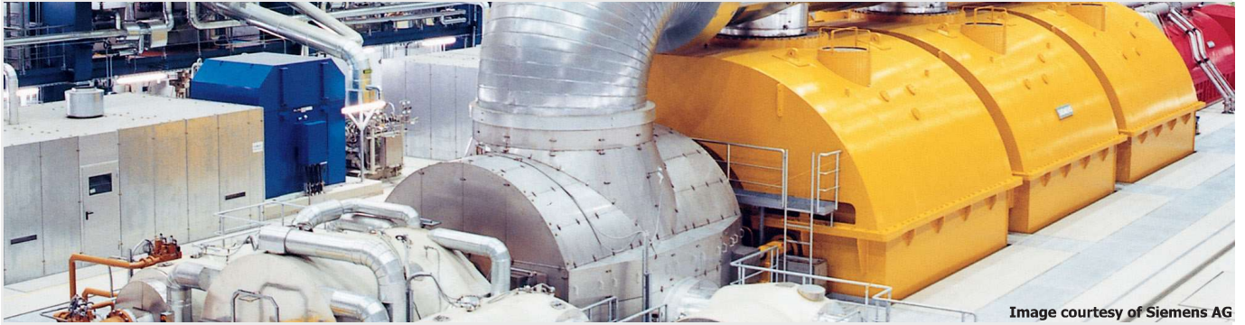
Image courtesy of Siemens AG
